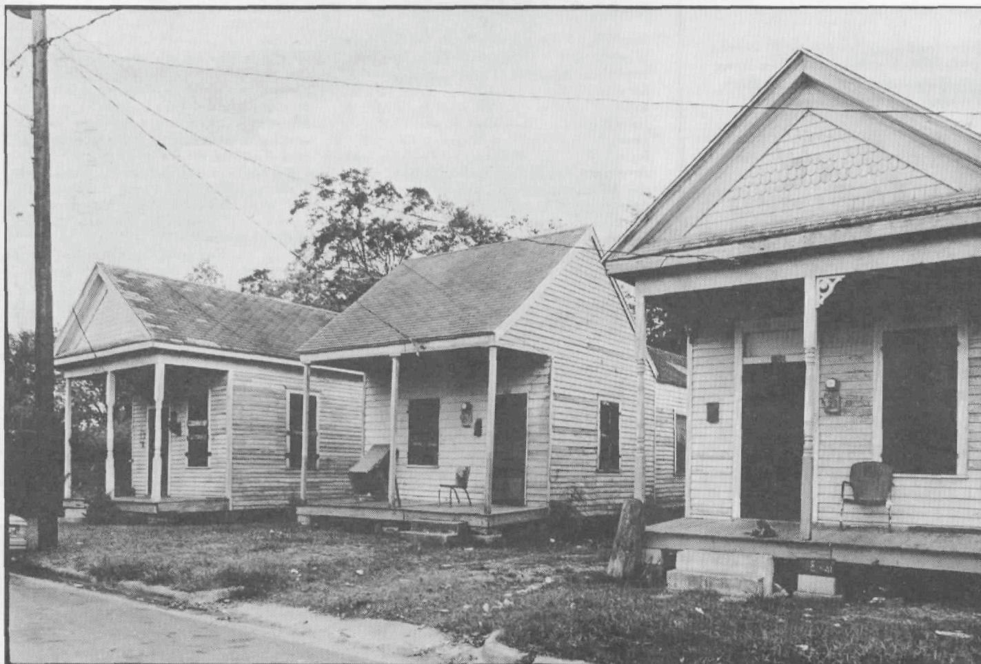
House on Robin Street. Preservation consultant Ellen Beasley believes that this may be the oldest house in Freedman's Town (Photo by Paul Hester)
