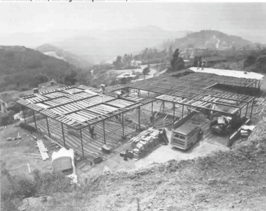
Below: Julius Shulman house and studio under construction, 1949, Los Angeles. Raphael Soriano, architect.
