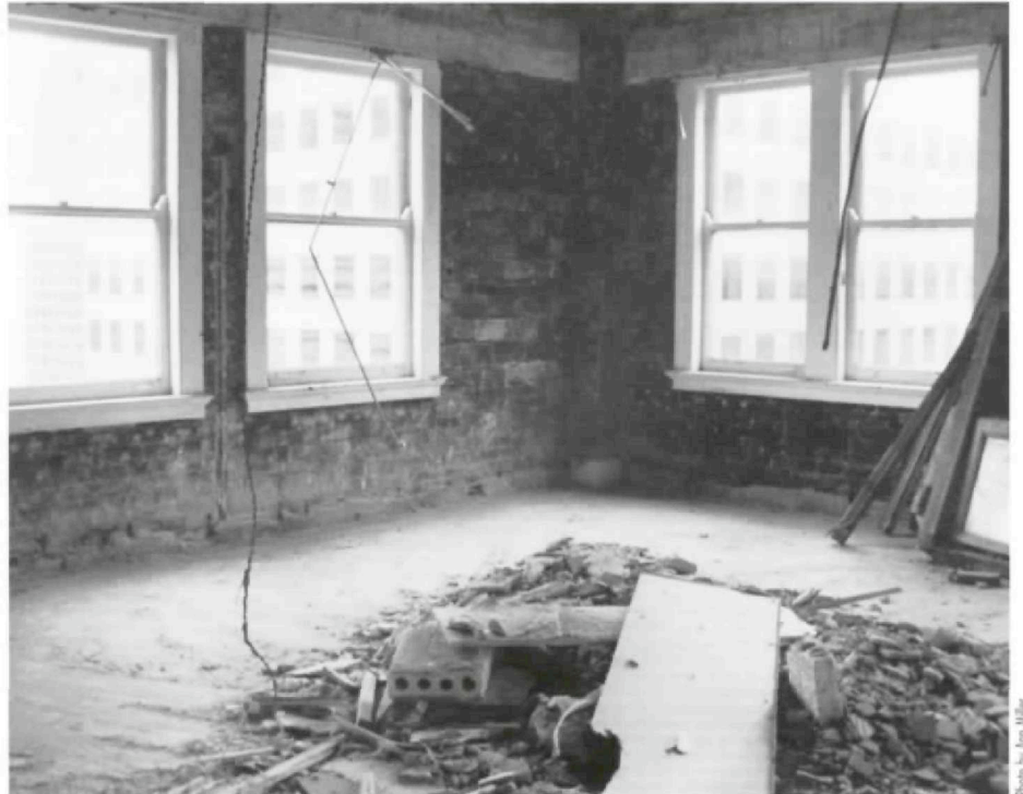
Before: To prepare for renovation into lofts, the upper floors of the Rice Hotel were stripped down to their bare walls.
