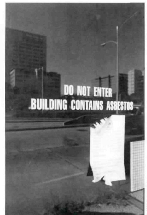
Adams Petroleum Center, entrance. Asbestos is a serious obstacle to refurbishing mid-century buildings.
