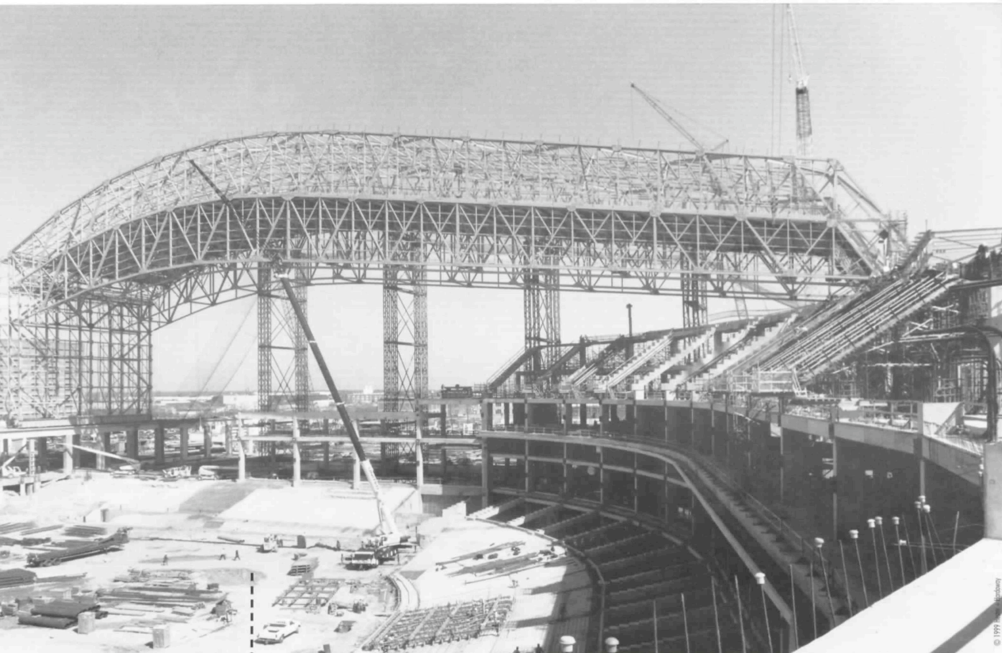
When completed, the retractable roof of the Ballpark at Union Station will, at its highest point, rise 242 feet above the playing field — 38 feet higher than the highest point in the Astrodome.
