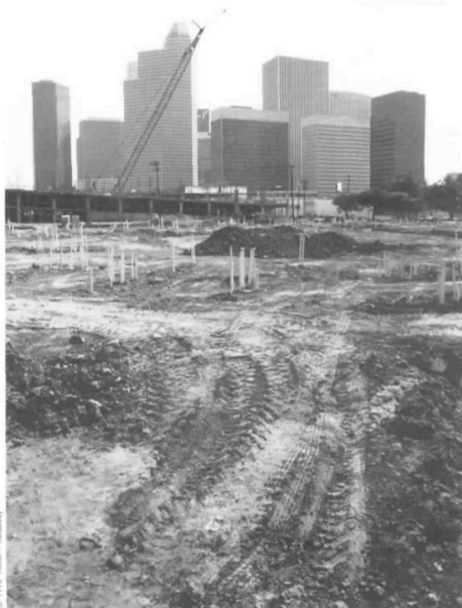
© 1998 Howe + Howbery Clearing for new townhouse and apartment construction southwest of downtown.
