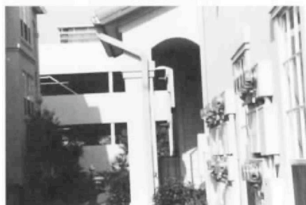
Electric meters at the Reata.
